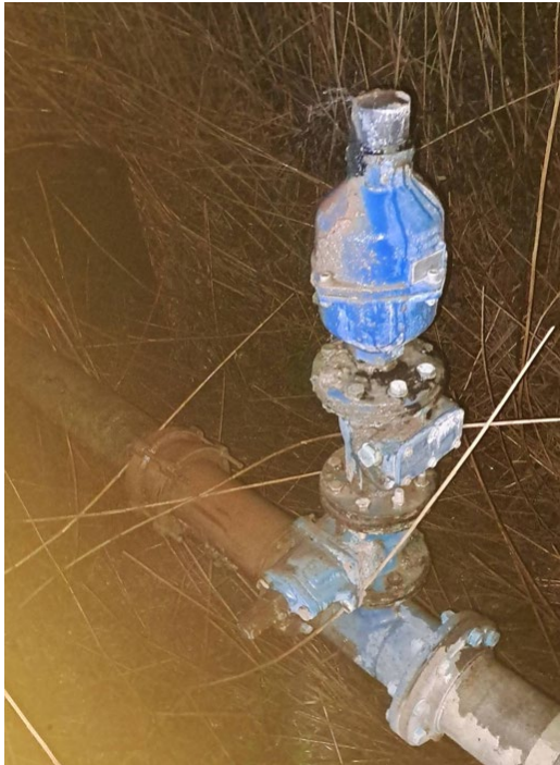
Leaking air valve
